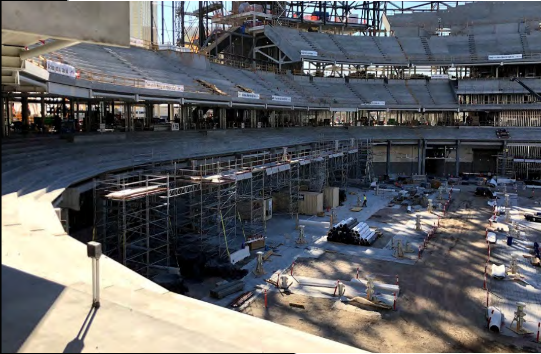
Above: Freyssinet cablenet prep work is underway in the bowl. Below: Field tray rail grade beam work continues under the south end longspan trusses.
